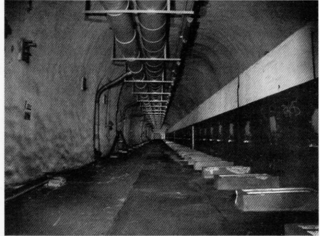
Battery room entrance (L on the plan).
